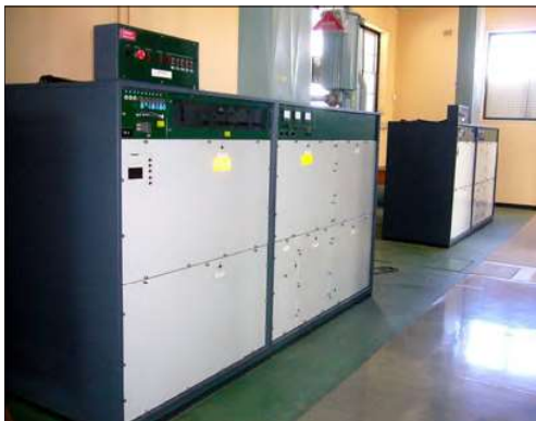
HF transmitter cabinets.
