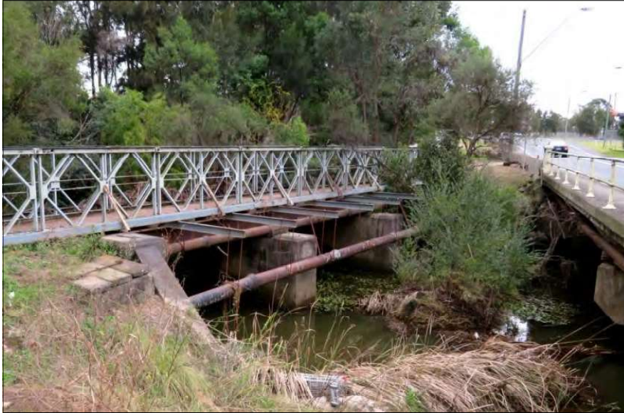
Harris Creek bridge. The water and sewer mains which it carries were probably its salvation, as it is unlikely to have carried a train since 1930. A Bailey bridge deck has been added to convert it to a footpath. The road on the right is Heathcote Road, planned for an upgrade. Photo: John Oakes.
