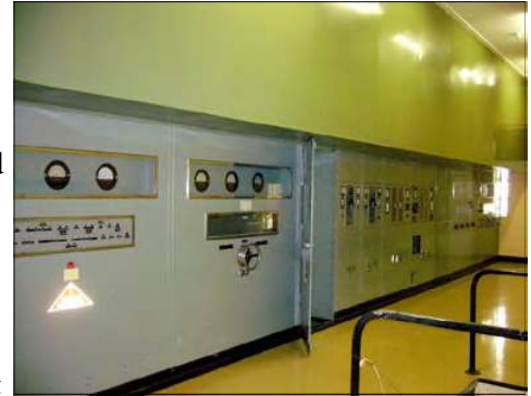
LF Transmitter cabinets.
