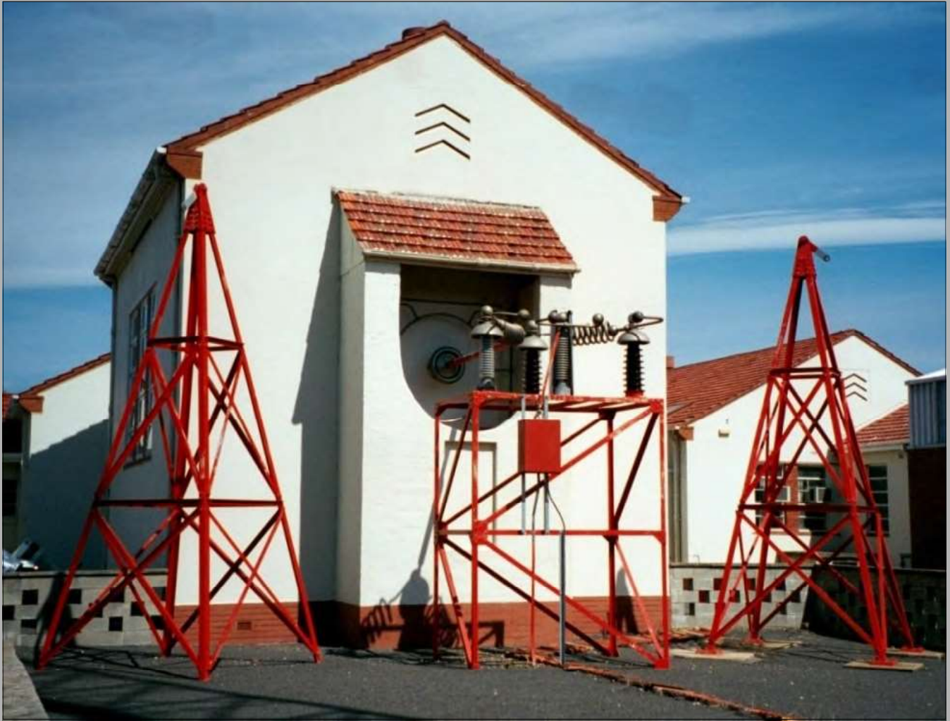
Belconnen Naval Transmitter Station, Canberra. Decommissioned Helix Room and feed supports to former LF Transmitter Aerial. Photo: Keith Baker.
