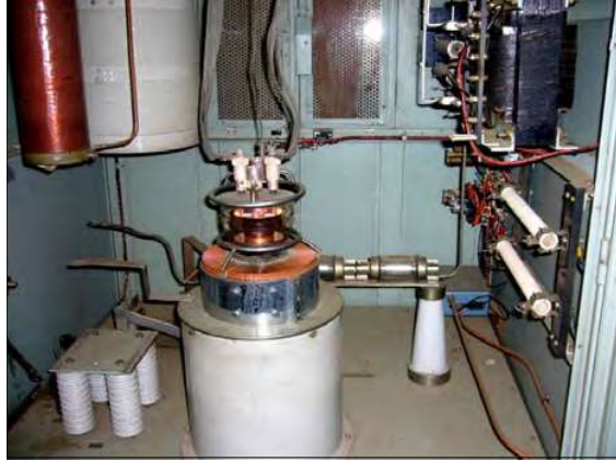
Air cooled valve in transmitter cabinet.
