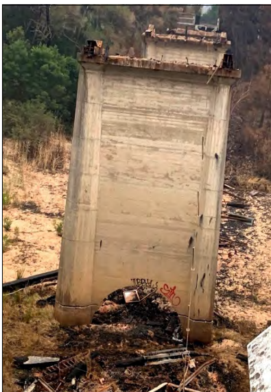
Genoa River bridge, showing cracks in the base of a leaning concrete pier, 2011. Source: East Gipps. Shire Council.
