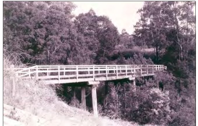
Bete Bolong Creek bridge, Bete Bolong, undated but probably c1997. Source: National Trust (Vic).
