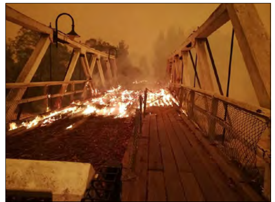
Genoa River bridge with decking on fire, 31 December 2019. Source: ABC Gippsland website.
