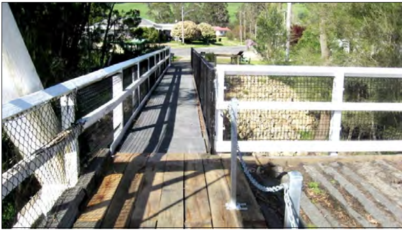
The township end of the Genoa bridge, showing the new narrow steel-decked pedestrian gangway across the failed timber abutments. In the foreground, a short part of the strip of new longitudinal decking is chained off from the old, probably unsafe, decking timbers. Source: H.Martin.
