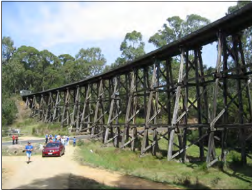
O'Grady's Creek rail bridge, structure from western end, Wairewa, 2009. Source: H. Martin.
