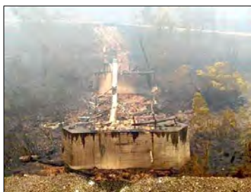
The Murrindal River bridge after the fire, January 2020. Source: EGSC.
