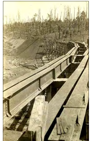
O'Grady's Creek rail bridge under construction, 1914-15. Source: Charles H Perrin collection - Vic. Railways - Museum Victoria
