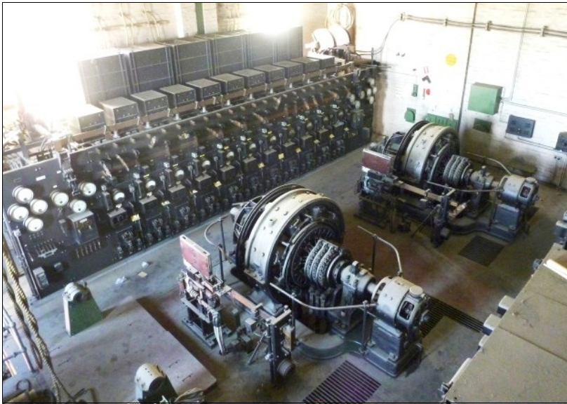
The interior of the former Malvern tramway substation, showing the two 1000kW rotary converters and the open panel DC Switchboard. Photo - Miles Pierce.
