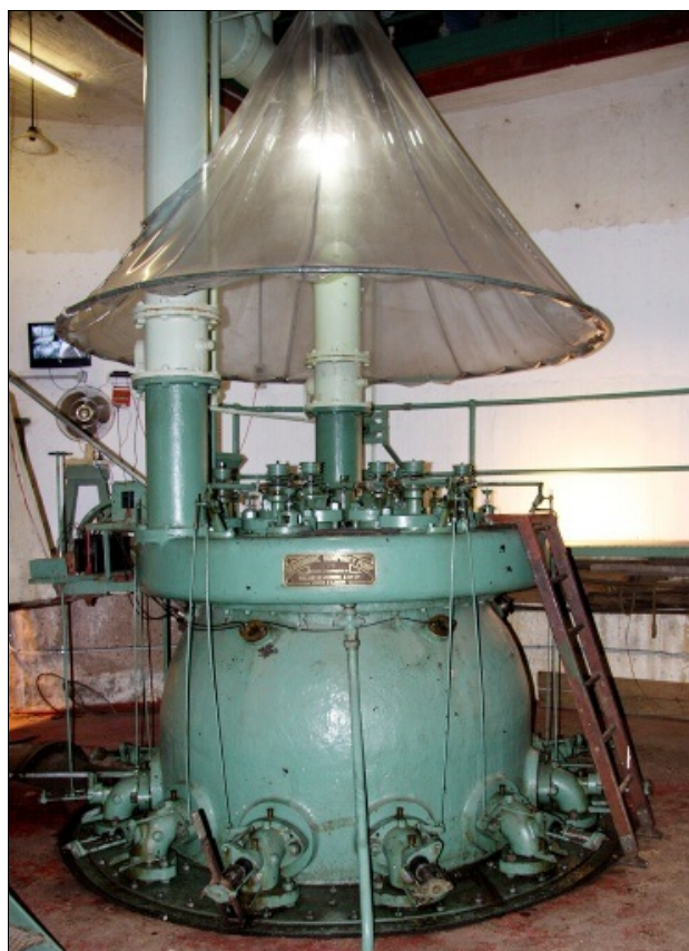
Humphrey Pump combustion head with gas hood. Photo R. Venus. Note: The gas hoods collect lighter-than-air combustion products – including the carbon monoxide which caused the problem in 2012 – and a fan draws them away from the operating floor (presumably vented through the roof – we're not entirely sure) Originally canvas, they were replaced with the clear material (probably a PVC) so visitors on the upper level could see the valves operating. – RV.
