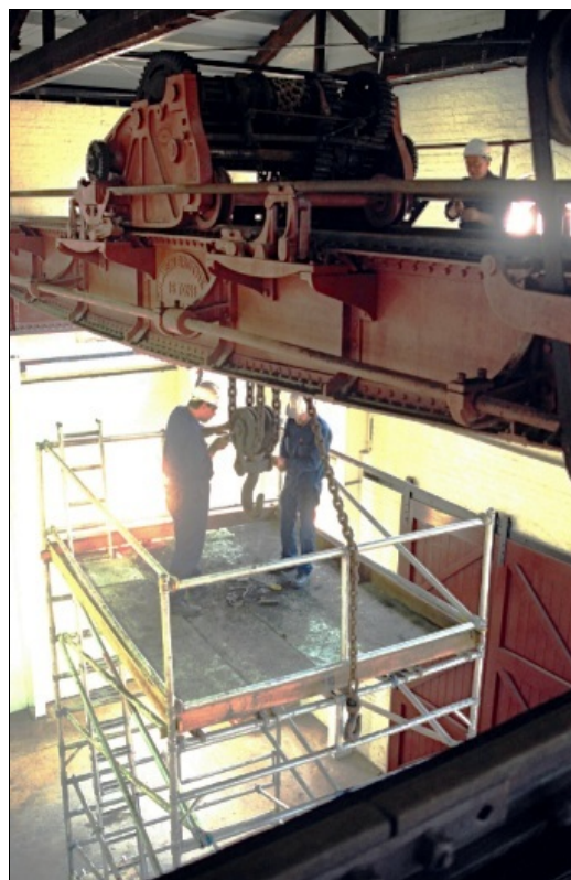
Engineers working on the restoration of the Craven Bros. Crane in 1995. Photo Carl Doring.
